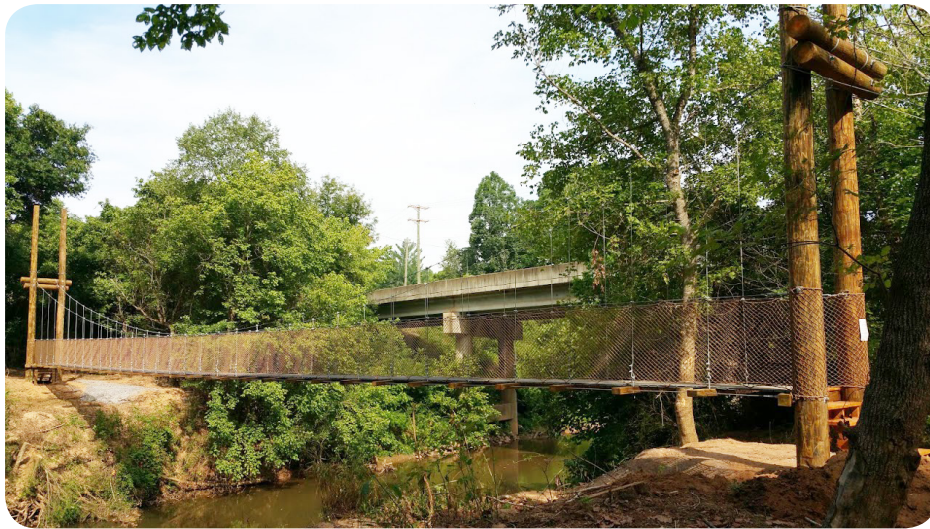
FIGURE 5.5.: Pedestrian bridge under construction for the Carolina Thread Trail that crosses the First Broad River and a portion of the trail. With the completion of this bridge, there is an opportunity to expand the Carolina Thread Trail west of Shelby through the Polkville Road Interchange study area.
