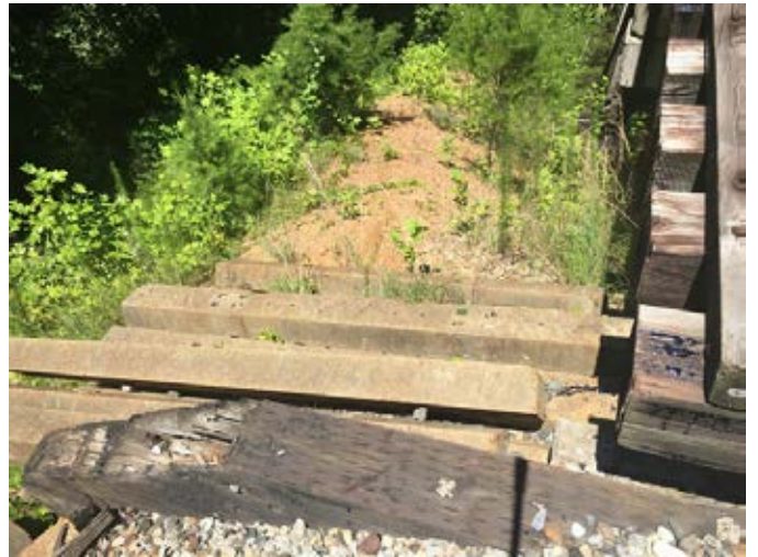
Debris at second rail trestle bridge.
