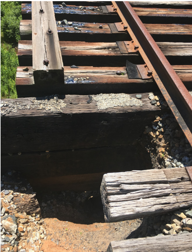
Scouring at second rail trestle bridge.
