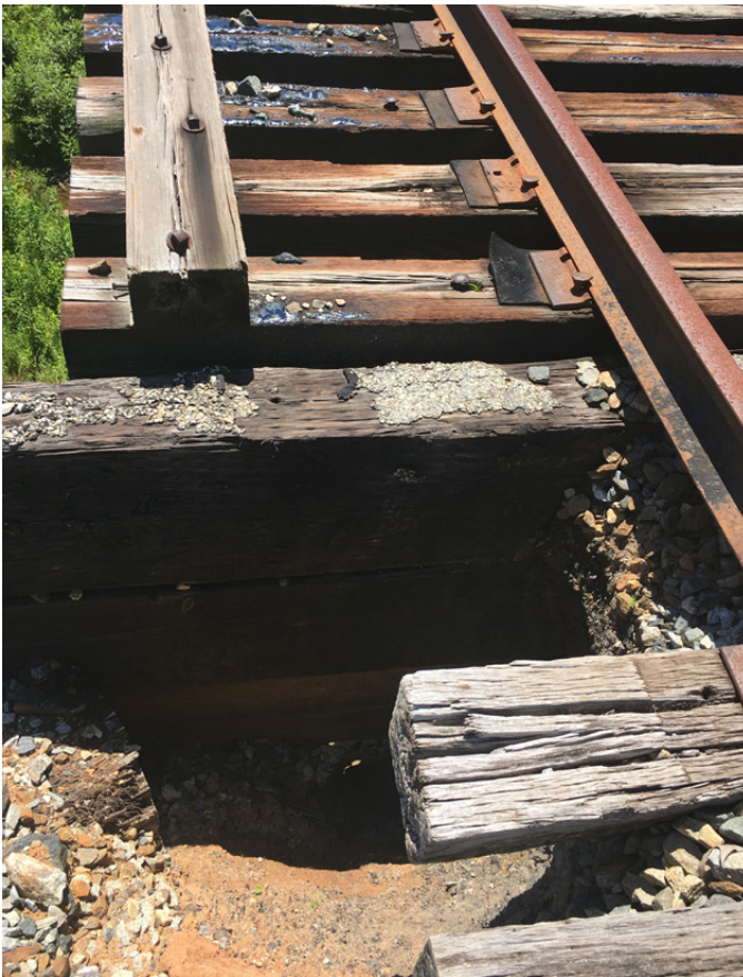
Scouring at second rail trestle bridge.
