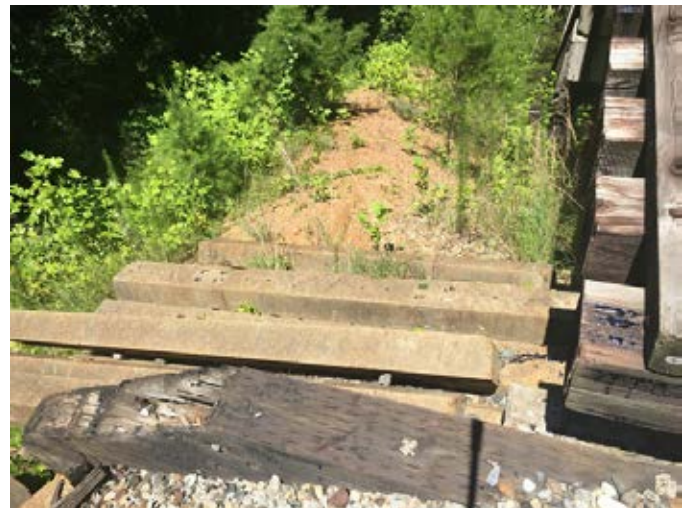
Debris at second rail trestle bridge.
