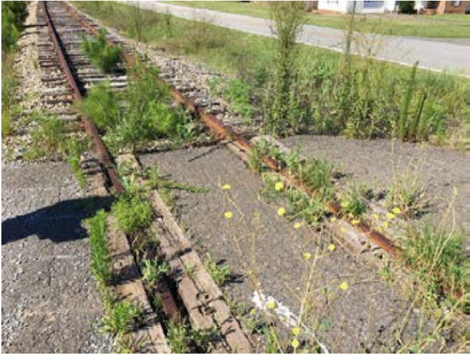
Existing conditions at driveway crossing.
