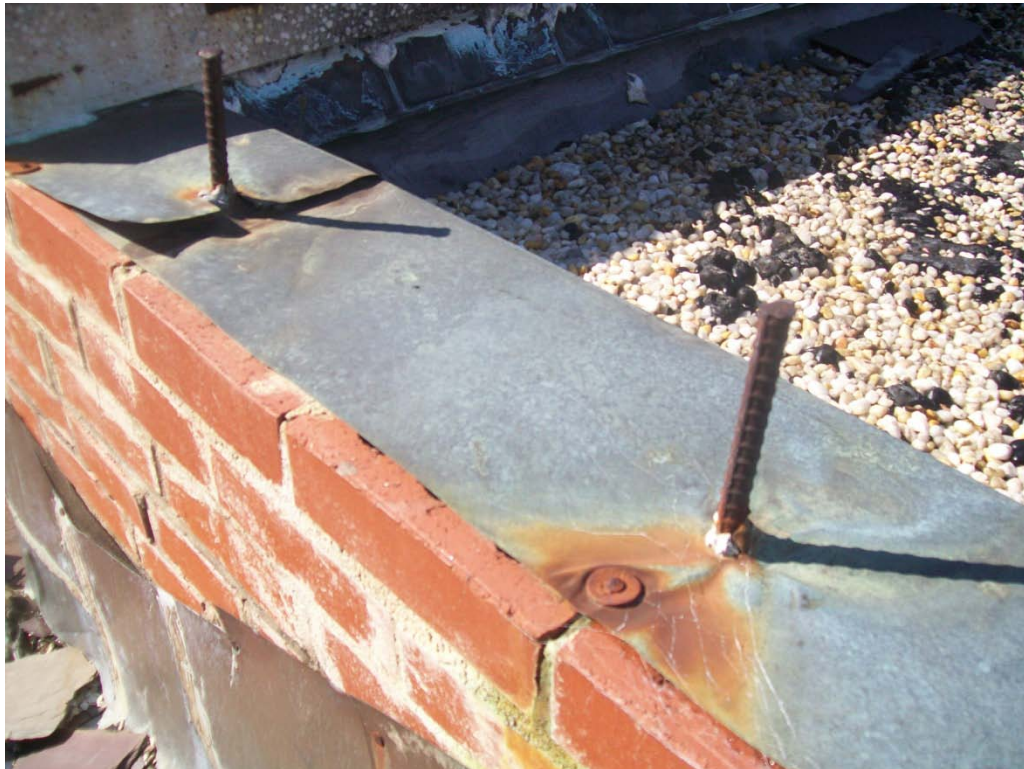
Photo 20: Area E - Missing Cast Stone Coping and Open Flashing
