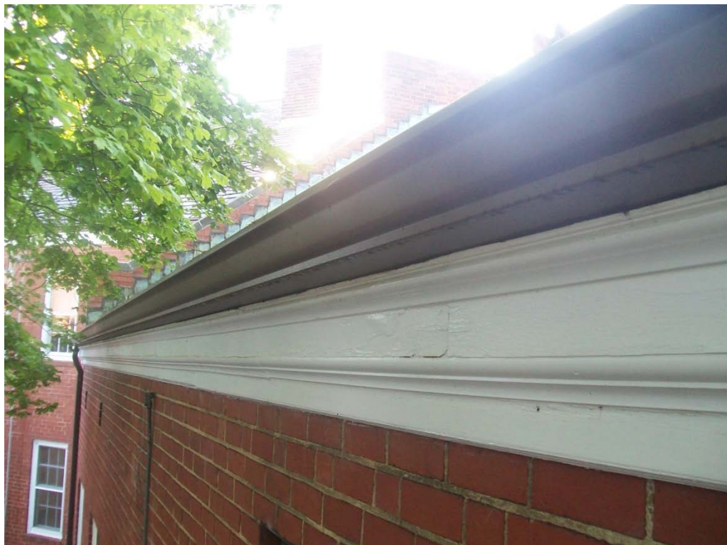
Photo 36: Typical Wood Fascia/Cornice Condition
