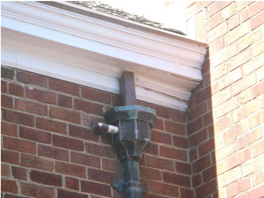
Photo 35: Wood Fascia/Cornice Condition Damage (Minimal Throughout)
