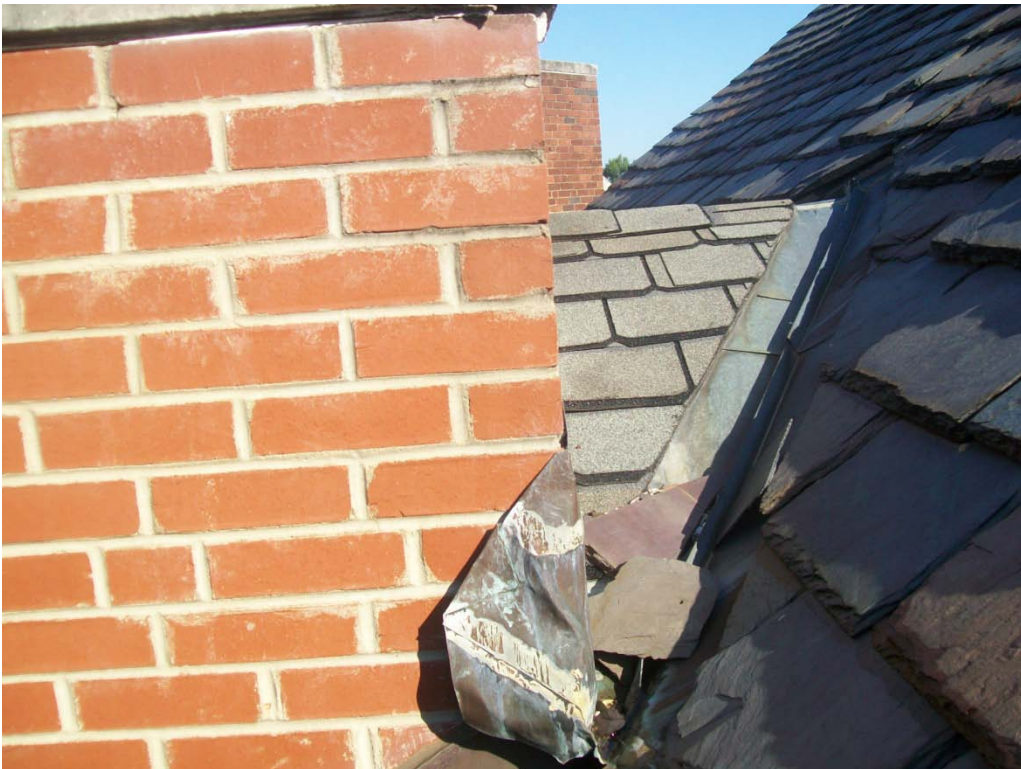
Photo 14: Open Cricket/Flashing Condition at Area C to Area E connection
