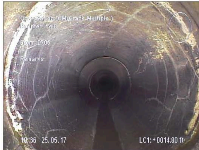
Date: 2017/05/25 Distance: 14.8 Ft Obs: Crack Multiple Comments:
