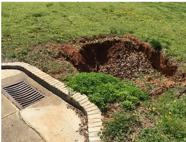
Poplar Circle Project Before Repairs
