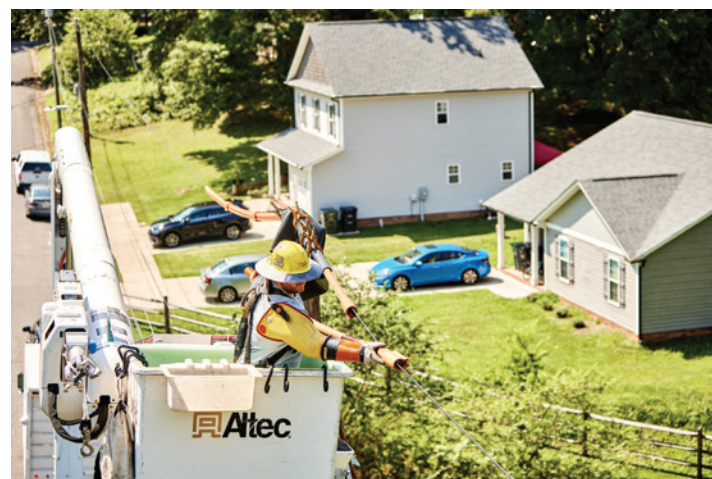
Top: Sharee Allen and her children McKenzie and Marc greet neighborhood lineworkers Terry Morton and Blair Barrier. Bottom: Concord lineworker Tim Furr works to repair an outage in a residential area.
