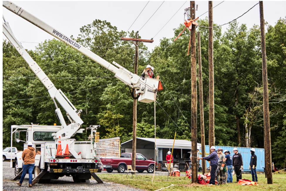
Students in SCC's Electrical Lineworker training program gain invaluable experience on the training ground.
